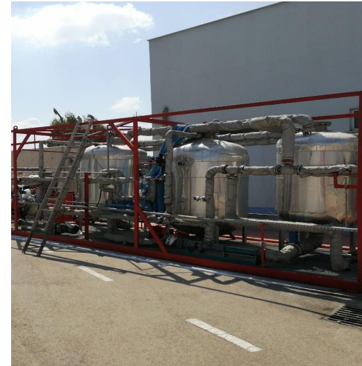
DEMO PLANT, TURKEY
